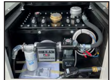
Diesel transfer pump setup
