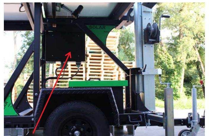
Weather proof control panel box.
